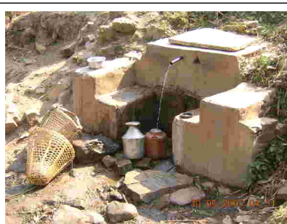
Outlet pipe from an 'open system' protected spring in a hill district in Nepal
